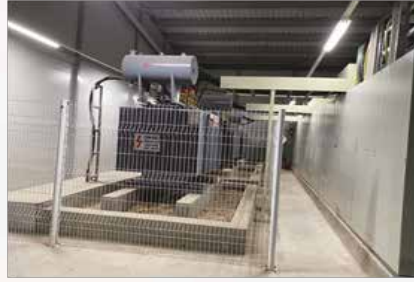
Oil/ Dry type Sub-Station
